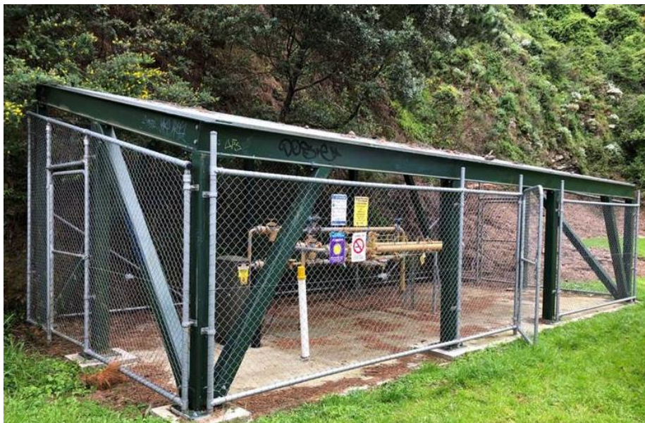
Figure 1: District Regulator Station, Wellington Town Belt
