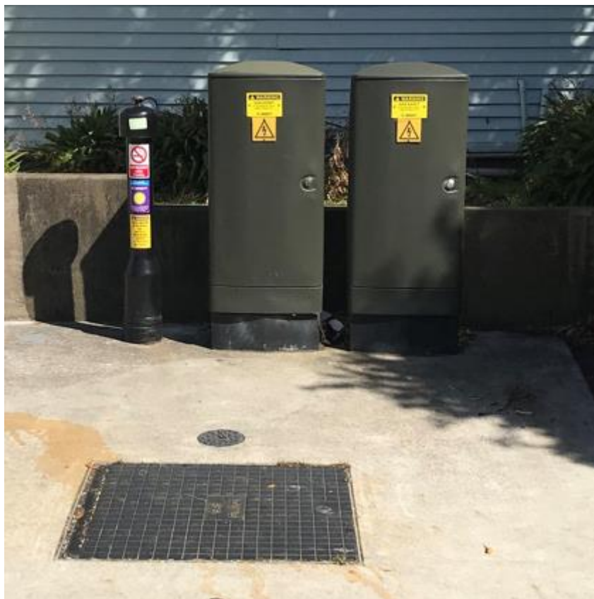
Figure 3: Powerco cabinets and SCADA equipment, 160 Tory St Wellington
