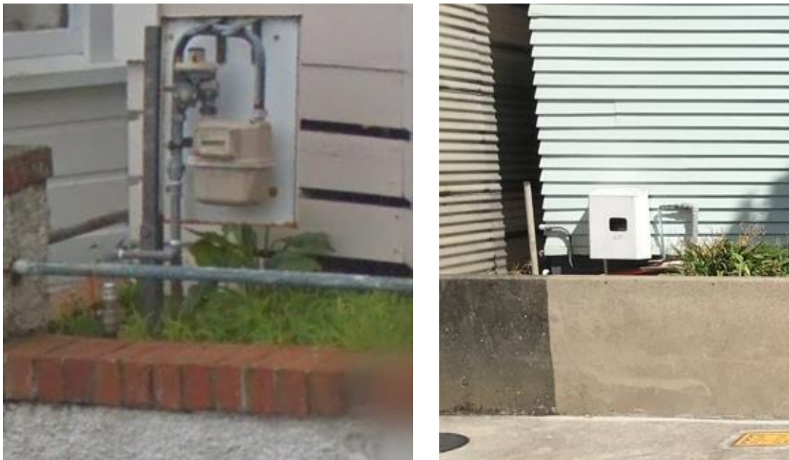
Figure 2: Photos of typical Powerco gas customer connection equipment
